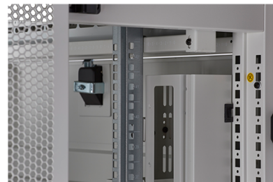
High-density vertical cable management
