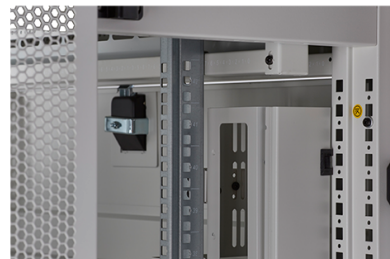
High-density vertical cable management
