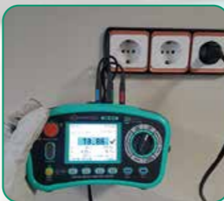
Loop test from a wall socket
